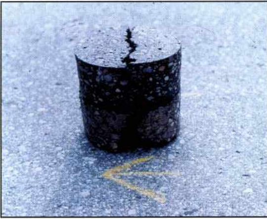
A core sample of 60mm asphaltic concrete on road base showing erosion at the interface of the road base and the asphalt, as well as in the road base material. This is caused by the ingress of water through the crack in the concrete.
