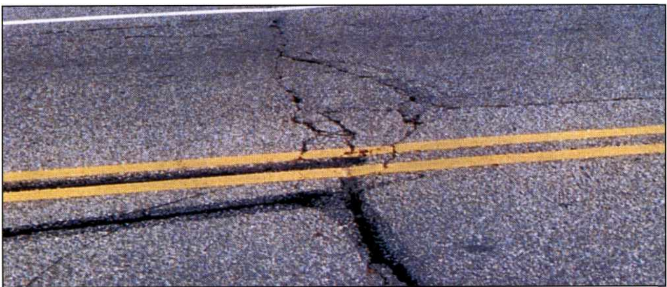
Half this transverse pavement crack has been crack sealed. As you can see on the far side, there is extensive transverse cracking and asphalt pavement deterioration where the crack sealing treatment was not carried out. The treated section on the near side has resisted further deterioration.
