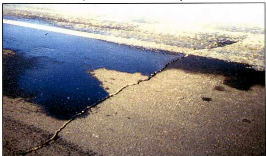
A transverse crack in this pavement was not sealed and has allowed water to enter the road base. Further deterioration will occur unless the crack is properly sealed as the ingress of water to the road base below will cause softening and pavement deflections leading to pavement failure.
