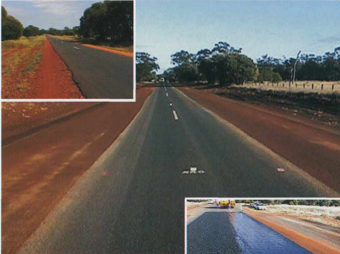
These photos show a section of Queensland DMR's Warrego Highway project in various stages of repair. The shoulders, weakened by constant wheel-path deformation and heavy rain, were in-situ stabilised and formation width was increased to 9.0m (centre photo). The SAMiflex E50 was able to be sprayed directly onto the prepared surface of the stabilised widened shoulders, eliminating the need for a primer seal.
