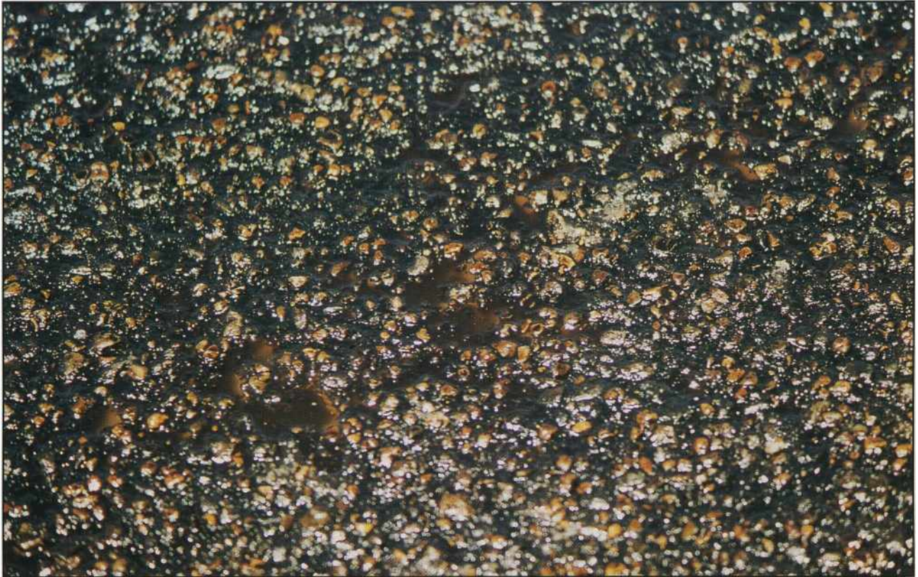
A close-up of Reclamite after spraying, showing it penetrating the existing spray sealed surface.
