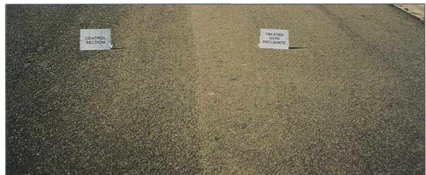
The difference between the quality of the surfaces on the Brigalow St control section (left) from the Reclamite "A" treated section is very noticeable.
