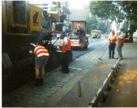
The new pavement is re-laid, neat to kerb and ready for traffic.
