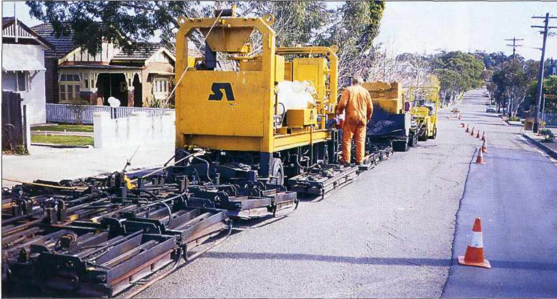
The banks of heaters in front of the HIPAR machine soften the asphalt in readiness for recycling.
