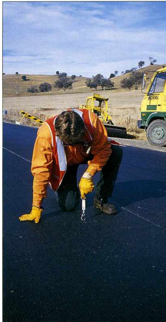
Checking that GlasGrid has properly bonded to the underlying AC layer prior to paving.
