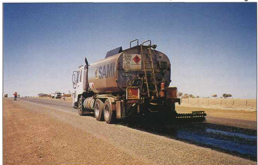
After being sprayed with Gilsabind "S", the existing polymer modified bitumen softened sufficiently to accept a new application of aggregate.
