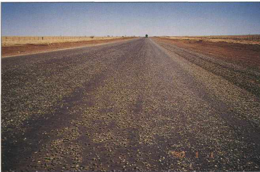
A 2 km long section of the Landsborough Highway in Central West Queensland had stripped badly and was even bare in places.
