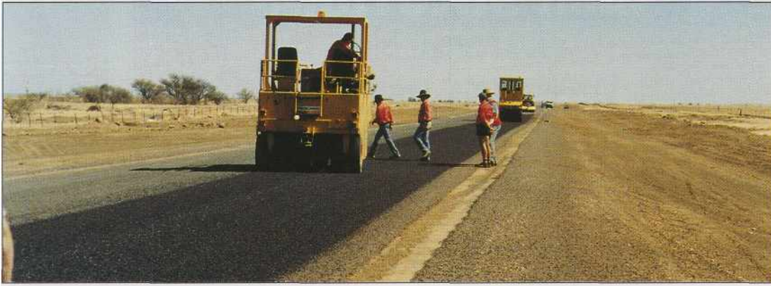
Queensland Transport's Alister Cullen said the Gilsabind "S" treatment had worked very well.
